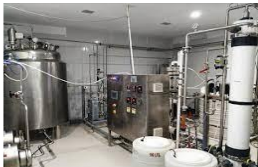
(Fig.-Pharmaceutical purified Water system)
